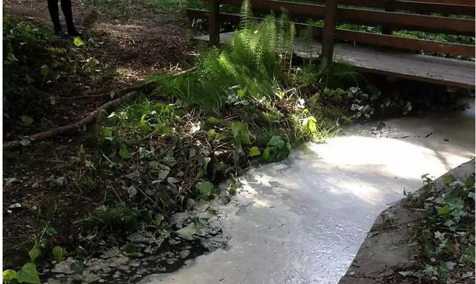
Concrete that has spilled into Glen Echo Creek during a pipe retrofit project by the East Bay Municipal Utilities District in 2015
